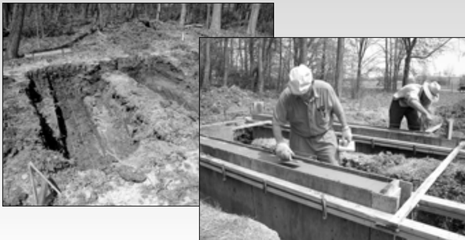
The photos above show the progress being made in the Sawmill foundation. At left is the groundwork completed and ready for the pouring of concrete. At right the poured concrete is being trowled to perfection.
