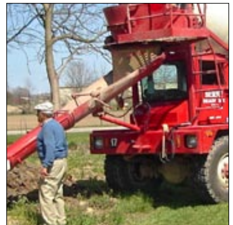
Kent V. Sprunger, project engineer, overseeing the pouring of the saw mill foundation
